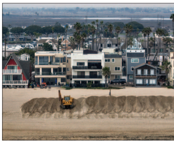
A heavy equipment operator builds a sand berm at Surfside in Seal Beach on Monday ahead of a strong storm forecast to arrive by the late evening.
